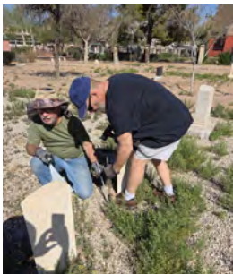
(L) Brothers Booth CC and Hoffay DC installed stakes for the GAR markers at Pioneer Cemetery in March 2026
